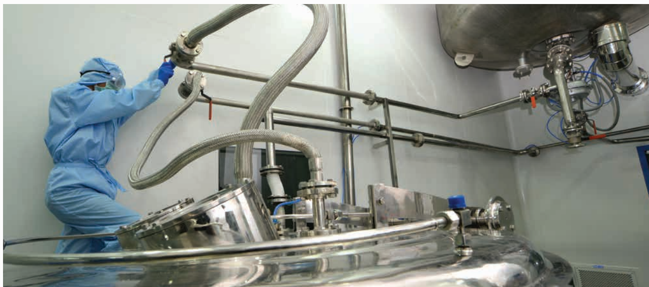
Isolation of products at our Mangalore facility
